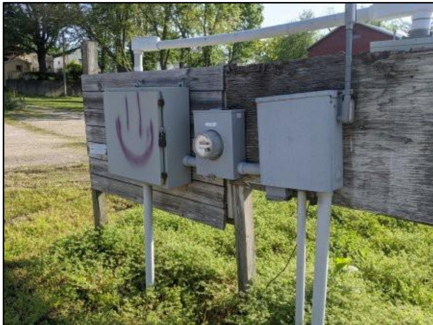
4: View of the electrical utility connections on the eastern portion of the property.
