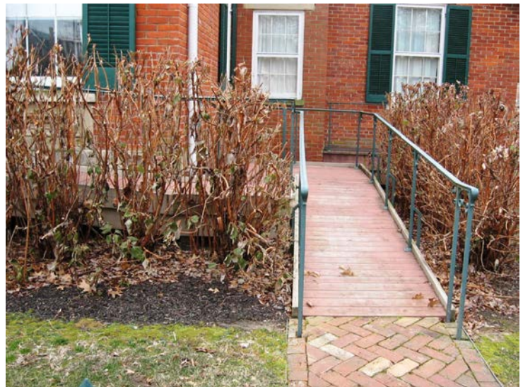
YES: At 301 W. First Street is an ADA ramp with a simple metal handrail and screened by landscaping.
